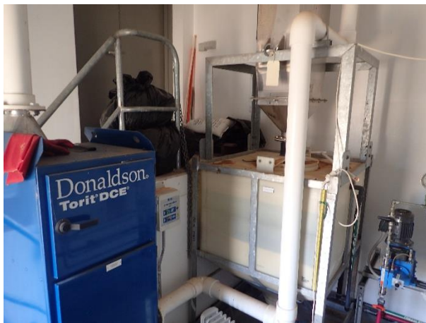
Sodium fluoride dosing system
