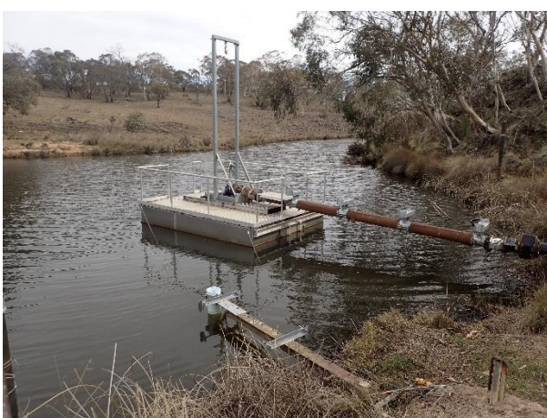
MacLaughlin River Water intake
