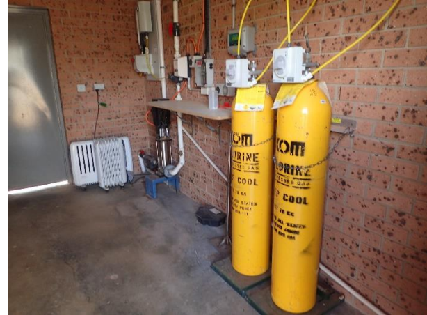
Chlorine gas dosing system
